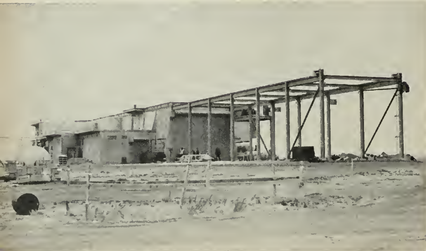
FIRST ATLAS launcher to be operational this spring has roof which slides off lengthwise. Unit of six is "soft."
