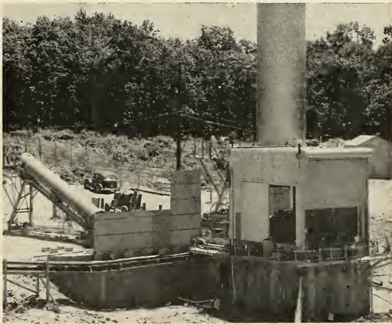
READY TO BEGIN static testing of the Pioneer rocket engine for the X-15 research aircraft is this new concrete and steel test stand built by Reaction Motors division of Thiokol Chemical Corp. The sloping tank (at left) is one of two propellant tanks which are an integral part of the stand. The large tank (background) is the division's 150,000 gallon water tank which supplies the entire test area.
