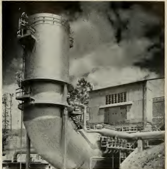
THIS "SCRUBBER" is part of the silencing and exhaust gas disposal system of the rocket engine static firing testing facility.
