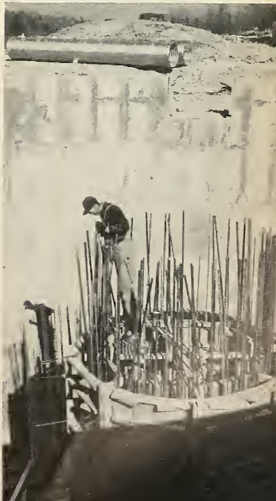
This pump shaft leads to underground receiving tanks at Rocketdyne's Neosho, Mo., plant. The company began moving in last month.
