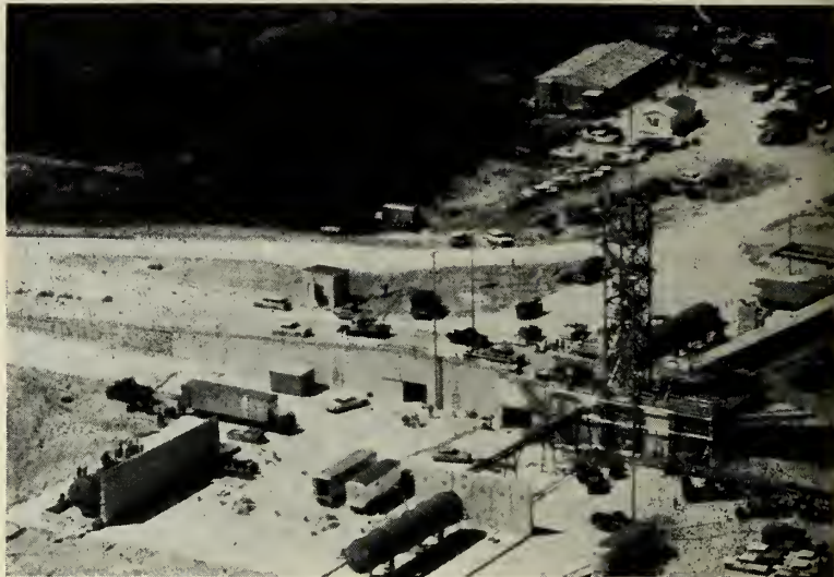
AERIAL VIEW of Complex 36 at Atlantic Missile Range, being built for launch of Centaur before mid-1961. Note the unusual right-angle flame deflector.
