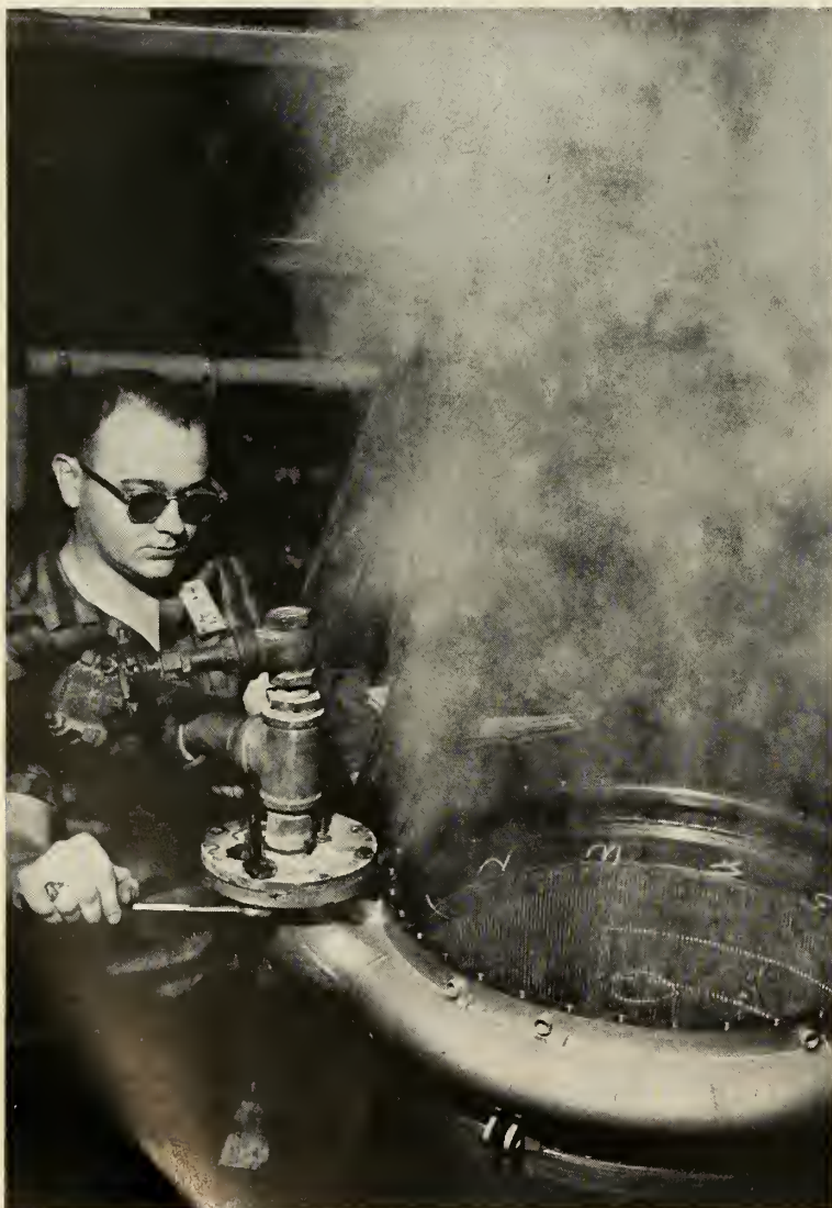
STEAM CLEANING of chamber is necessary to meet rigorous cleanliness requirements of Atlas engines. Workman tightens connection to chamber manifold,
