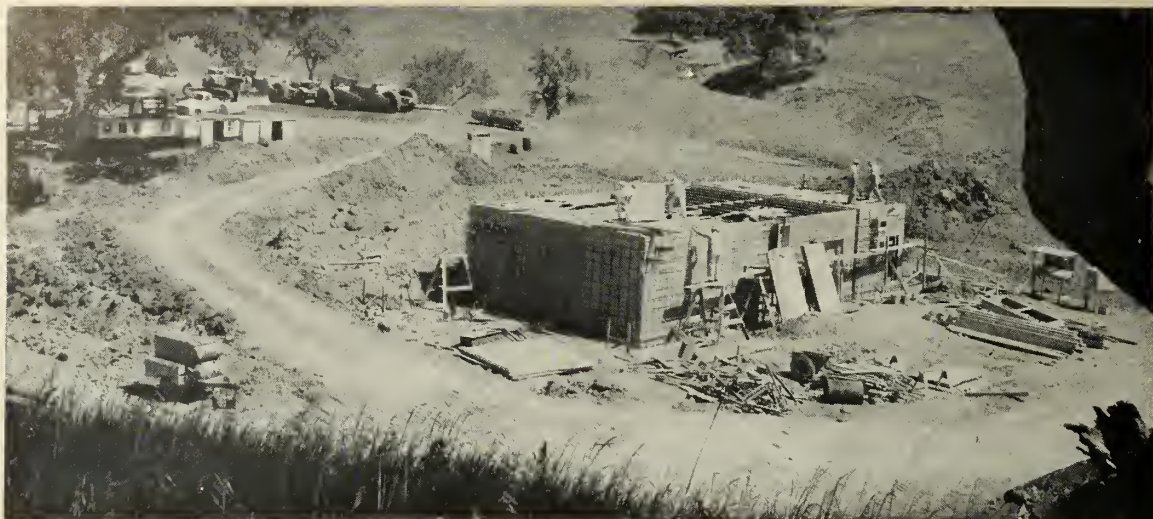
PROPELLANT mixing station with 200-gal. capacity goes up at UTC's Coyote Calif., center. Control center is at left.
