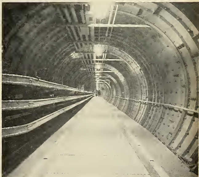
INTERIOR OF the 800-ft.-long access tunnel to Titan silo. Entire tunnel is lined with bolted, riveted and welded circular steel rings to guard against ground shock. The trays at the left carry instrumentation and other electrical cables to the silo from the control center. There are sub-tunnels for routing utilities to the missile.
