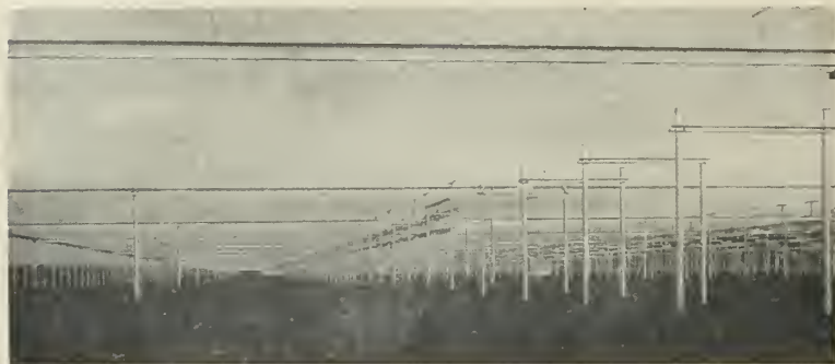
RECEIVING STATION antenna array is over a quarter-mile long and 300 feet wide.
