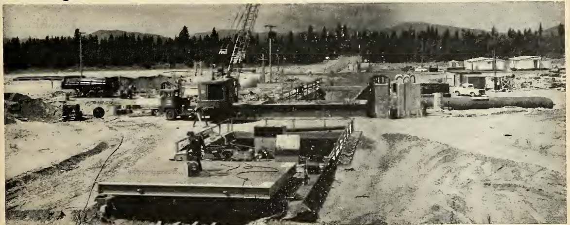
FIRST 'HOLLYWOOD HARD' Atlas pads are taking shape at Sheppard Air Force Base near Wichita Falls, Tex. Being con-
