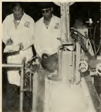
SIGMA welding is used by Reynolds Metals to make longitudinal weld on Redstone's center section.
