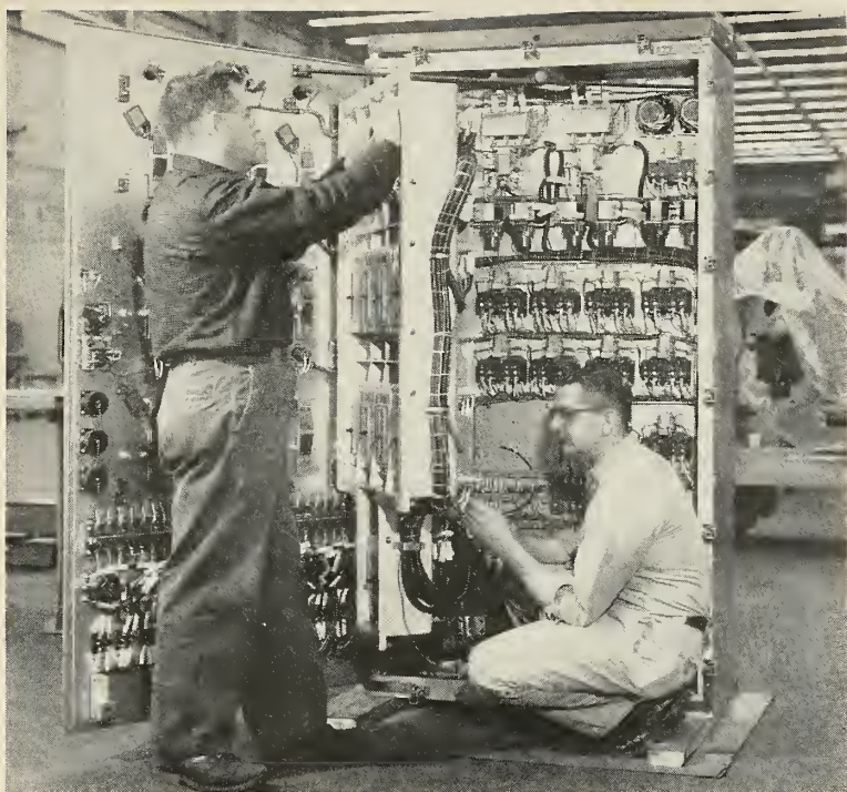
CONTROL cabinet for Talos launching system. Panel provides power distribution for launcher power drives, missile warm-up power and control power supply portions.
