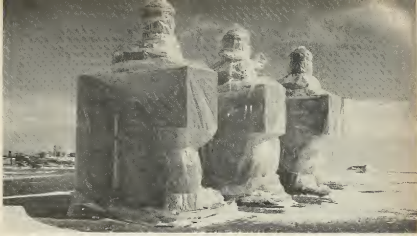
TRIO OF GIANT plastic-wrapped 1600 KW transformers stand on the Wyoming prairie prior to installation in an Atlas ICBM base. They symbolize enormous power requirements and vast quantities of special equipment needed by missiles.
