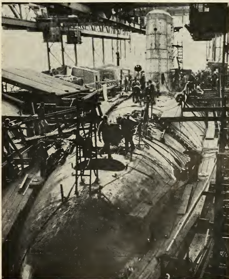
FIRST POLARIS submarine, George Washington, as she was being constructed in a record-breaking two-year period at Electric Boat.
