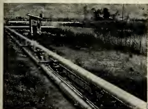
VACUUM-jacketed liquid hydrogen transfer line 2000 feet long connects Air Products' West Palm Beach, Fla., plant with a Pratt & Whitney test area. See report on liquid hydrogen, p. 21.
