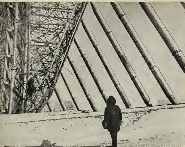
SOME 40 back stays and trusses each weighing seven tons are required to support surveillance radar at BMEWS Site I.
