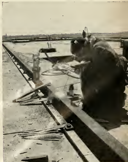
WELDER IS APPLYING finishing touches to the rails that will guide the huge servicing gantry handling the Atlas .
